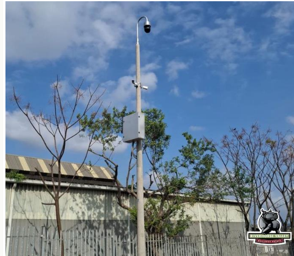
New CCTV camera infrastructure
